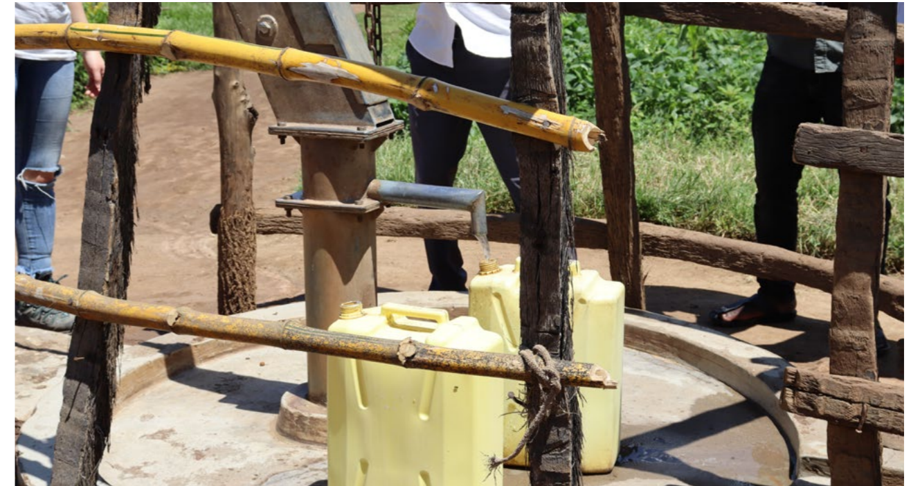
A team working on water boreholes, to provide fresh and clean water for a community in Uganda, with one of Canon Medical UK's CSR partners, CO2balance.
